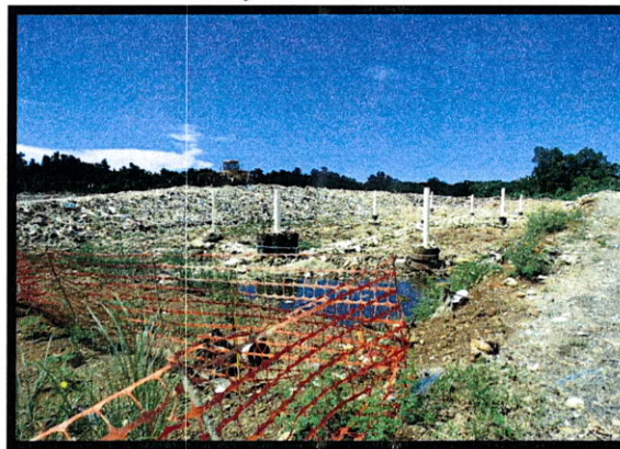
Photo 2: The newly semi-aerobic Dekehtik landfill
