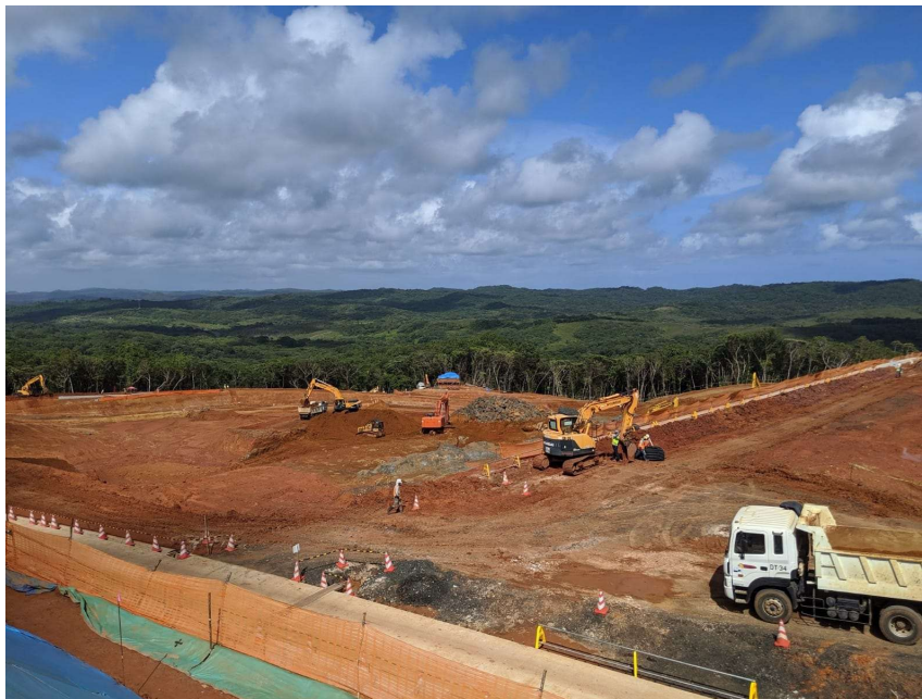
Figure 16: Construction underway at the national landfill in Aimeliik State. (UNEP Consultant team, November 2019)
